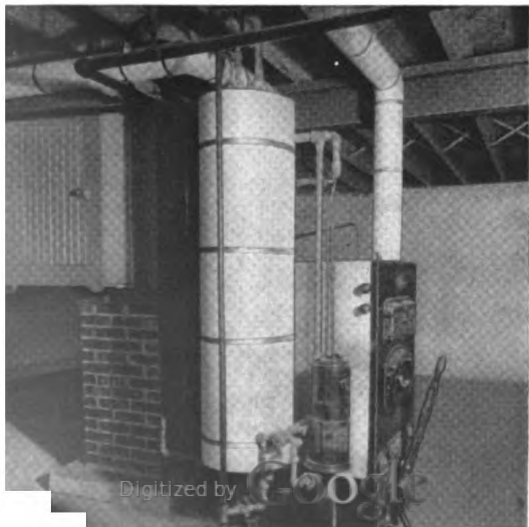
Asbestos tank and pipe coverings conserve household hot water supply.
